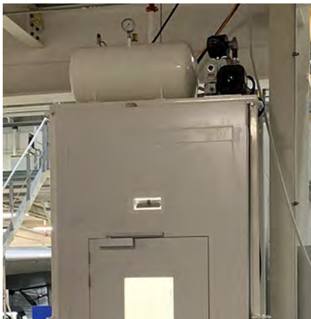
Here installed on top of entrance hall : a vacuum tank and a pump
